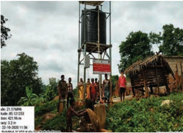
Solar operated drinking water supply point through convergence at Balidihi VSS, Barkote Range of Deogarh Division
